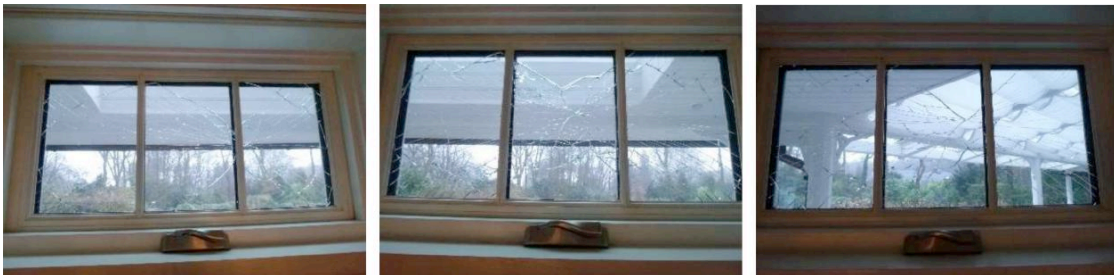
Photos 15, 16, 17: Three imploded units (numbered 1, 2 and 3) with broken inside panes. All are hinged vent windows situated right under the large canopy on the back side of the villa (photo 4).
