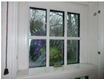
Photo 21: Imploded unit (numbered 7) with broken inside pane. Situated in a top sash window at the first floor bedroom in the SSE facing (back side) façade.
