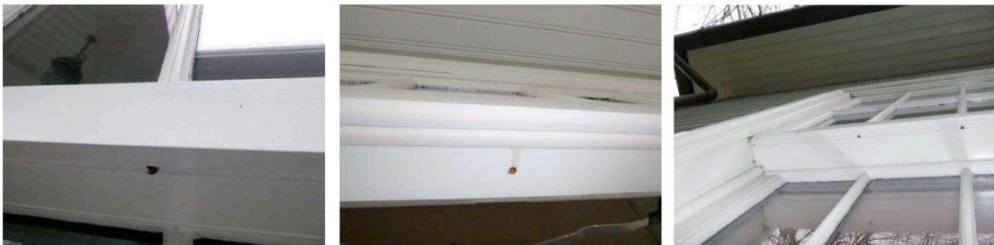
Photos 10, 11, 12: 1-3 weep holes for water drainage per window.
