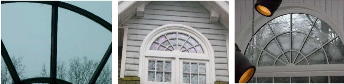
Photos 28, 29, 30: Signs of touching foils and or glass panes inside the cavity: Moiré, interference discoloration and inside condensation.
