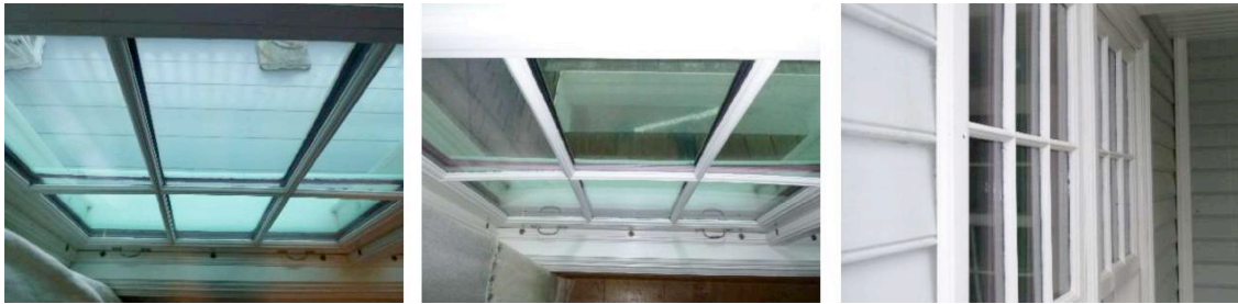
Photos 22, 23, 24: Concave shaped glass panes, clearly visible by the bent crossbars..
